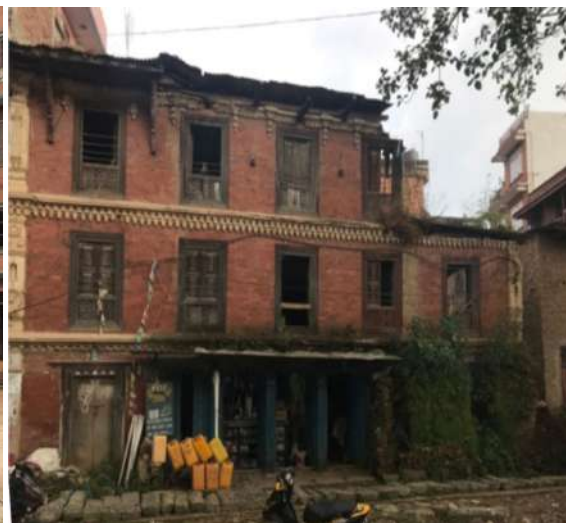
Figure 14: Partly collapsed building (2021). Source: Padma Sundar Maharjan.
